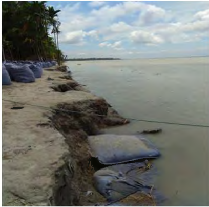
2. a) Bank erosion
