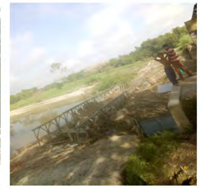
6. l) Collapsed bridge
