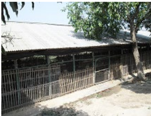
E Absence of boundary wall at Baghmara
