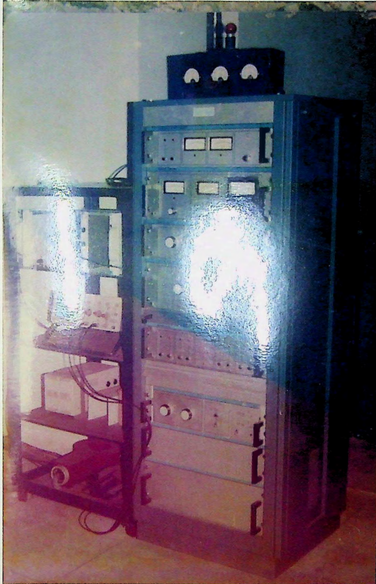
Fig.2.3 Partial view of the remote control console of the neutron generator.
